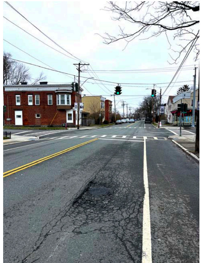
▲ Pavement condition along 3rd Avenue in the City of Watervliet.
