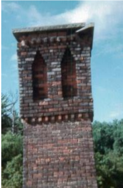
Valley Paper Mill Chimney Capital 5ft Square x 6 1/2 ft High (photo 2012 before dismantled)
