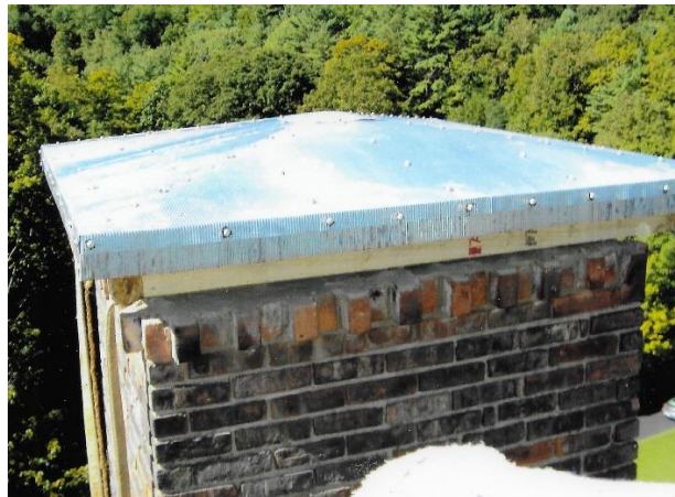
Valley Paper Mill Chimney Capped To Mitigate Further Deterioration (photo 2012 after capital removed) (current today 8/30/2024)
